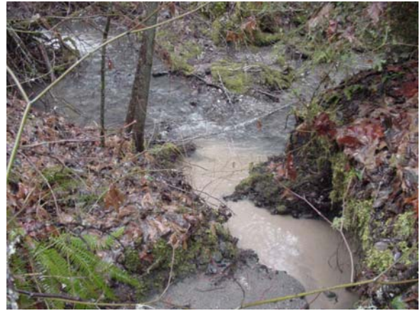
Fig 47 Erosion on side of road continues to down into Spring Creek mixing with clear water
