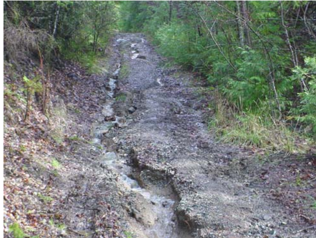
Fig. 8. Upper East Fork Road erosion damage from one year
