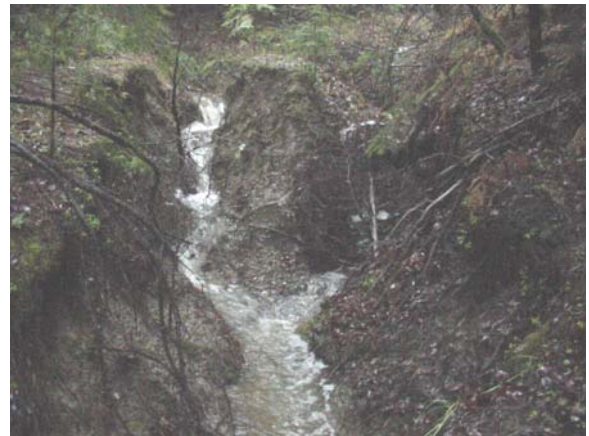
Fig 49. Runoff travels down road and enters gully during rainstorm continuing erosion
