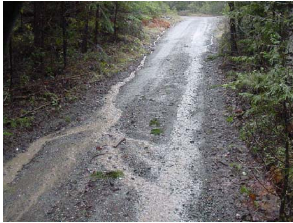
Fig. 44. Erosion down steep forest road carries fine material downslope
