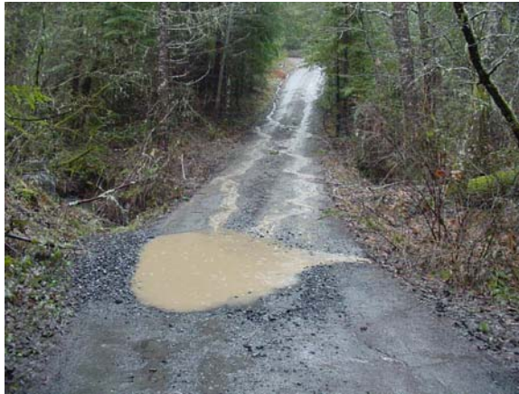
Fig. 45 Erosion on Spring Creek Driveway collecting at crossing of Spring Creek
