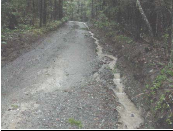
Fig 50. Erosion along side of road continues to cut ditches and removes gravel to Spring Creek
