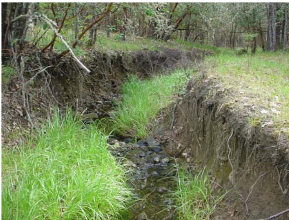
Gullies formed along Lower East Fork Road by cross-drained culvert outflow
