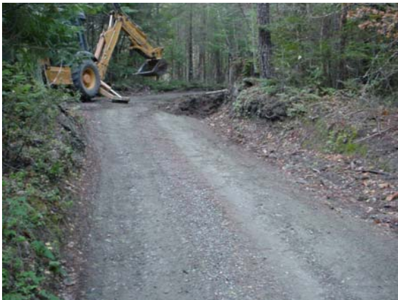
Fig 51 Road repair began with knocking down the berm and filling in the ditches
